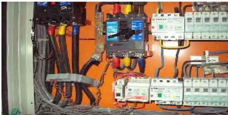
Figure 9: industrial main switch
